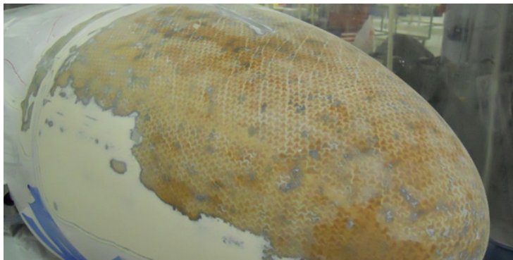
Stress lines remain visible on a composite surface after existing paint and primer are removed.
